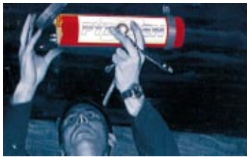
Simply installed close to the potential hazard
